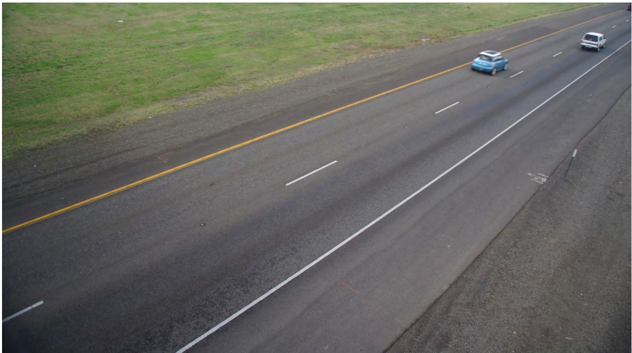
Surface was paved in 2007, picture taken in 2010. Note wear in the wheelpaths of outside lane.
