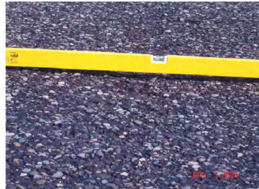
Figure 2.13: Studded tire wear on I-5 MP 303.75 SB in Oregon
