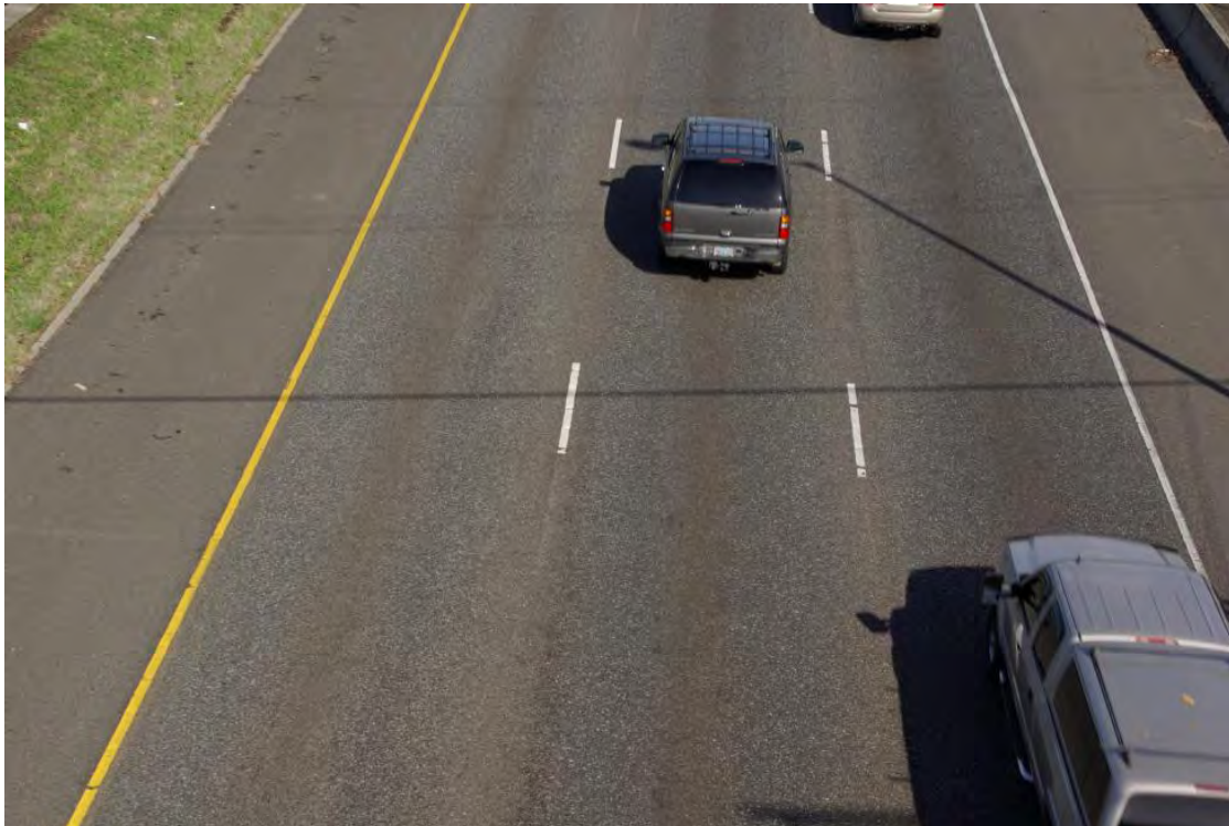
Surface was paved in 2005, picture taken in 2010. Note wear in the wheelpaths of all lanes.
