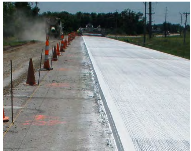
The Oak Crest Hill Road $1.845 million stimulus job is a concrete overlay that covered two lanes and spanned nearly 5.5 miles from start to finish. The road was widened to provide an extra lane for bicyclists.
